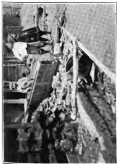
CLOGGED DRAIN ON MAURICE STREET
